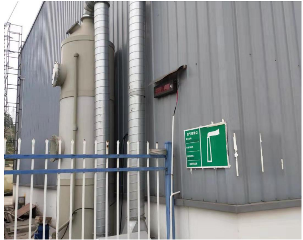
废气排放口标牌
